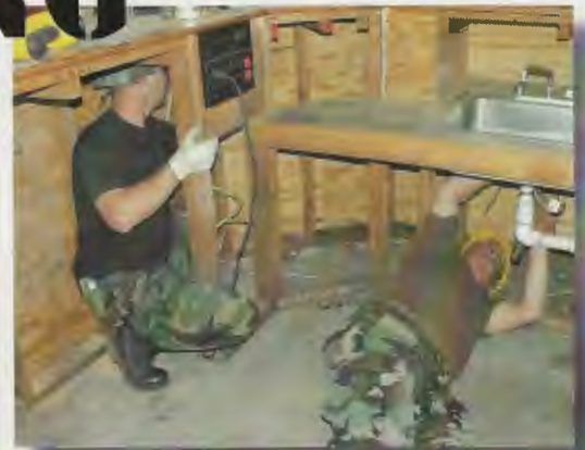
Staff Sgt. Soojin O and Master Sgt. Randy Aeschliman install a new plumbing fixture inside the Camp Morena Rec center.
